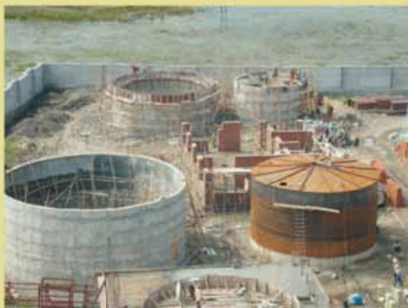
Co - Gen Water Treatment Plant
